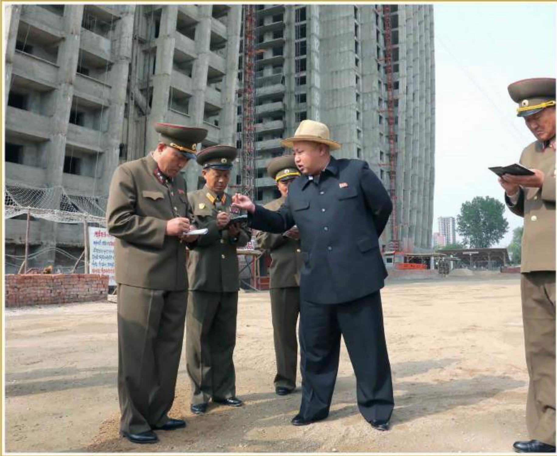
Kim Jong Un visits the construction site of apartment houses for teachers of Kim Chaek University of Technology in May Juche 103 (2014).
